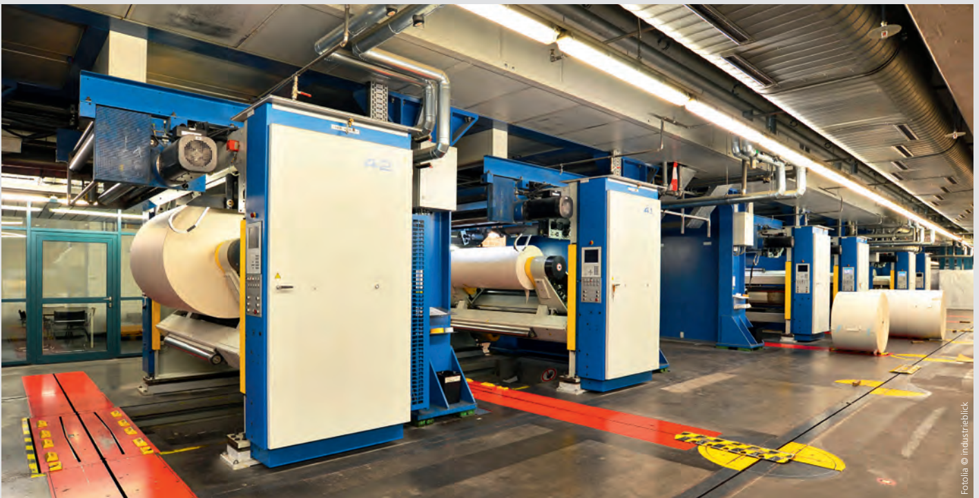
Object protection is installed for separate machining centres where fire flashover to other areas must be prevented.
